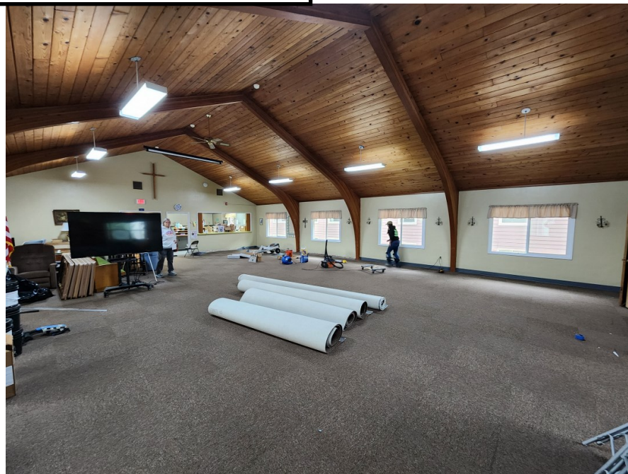
Finishing the face board in the Fellowship Hall after carpet was laid. Photo taken and submitted by Diane Hanson.
