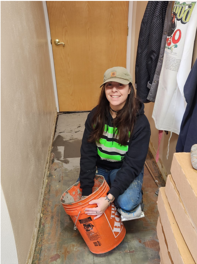
Sam, RES COM employee, works diligently in hallway to bathroom. Photo taken and submitted by Diane Hanson.
